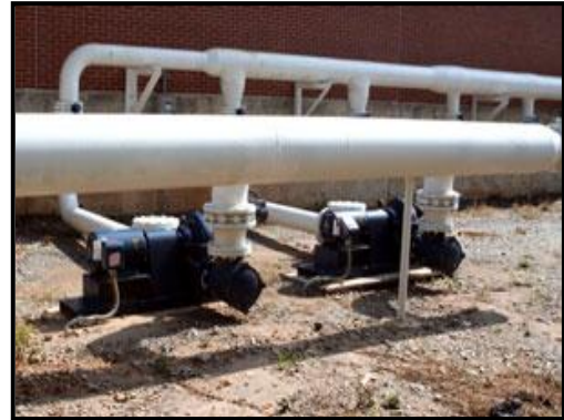
Water Pumps Fueling the A/C Units
