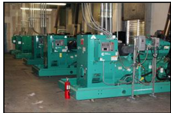
Backup Power Generators
