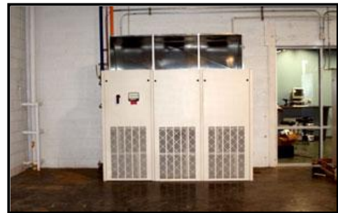
An A/C Unit Cooling the Server Area
